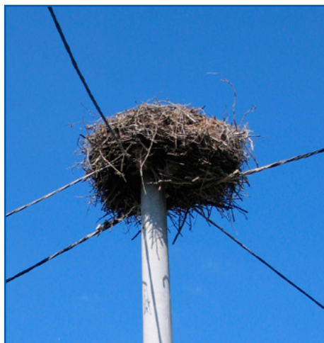
Nest on a modernized power line (wires in black insulation are braided). Photo: AT
