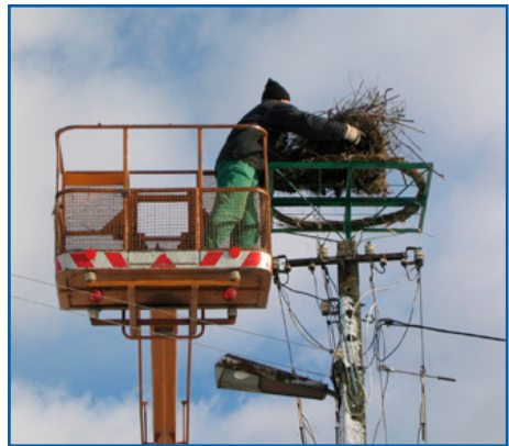
Inserting lining on a metal platform installed on a power pole. Photo: AT
